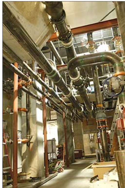
Photo courtesy of CDi Engineers Special low-velocity ducts in McCaw Hall restrict noise and enhance energy efficiency.
