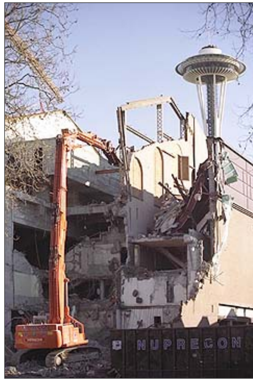
The long-reach tool on this modified Hitachi excavator helped demolition crews take apart the structure while preventing damage to nearby buildings and public areas.
