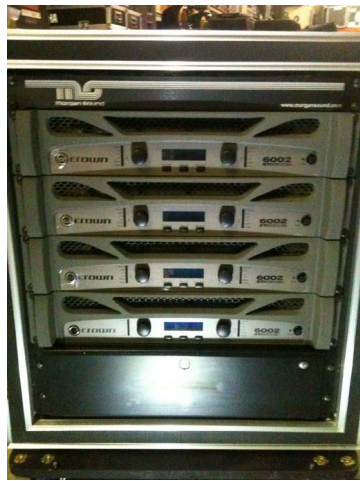
Custom amp rack with four Crown Mti 6002 amplifiers
