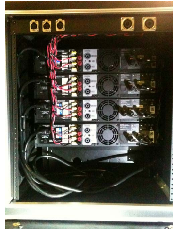
Rear of the custom amp rack. Not shown is a custom AC panel with L14-30 twistlok connector and rear-mounted 20-amp quad box.
