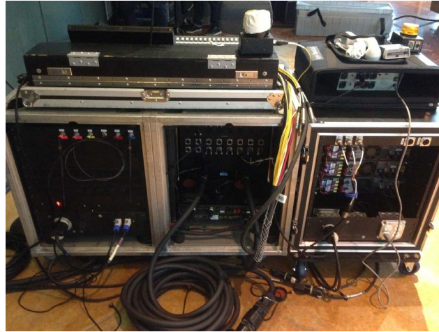
Rear view of the picture at the left of this one. In the amp rack at the right, you can see the custom AC panel with the L14-30 twistlok connector and the quad box.
